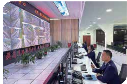
The Intelligent Operation and Management Platform of GDH Highway
