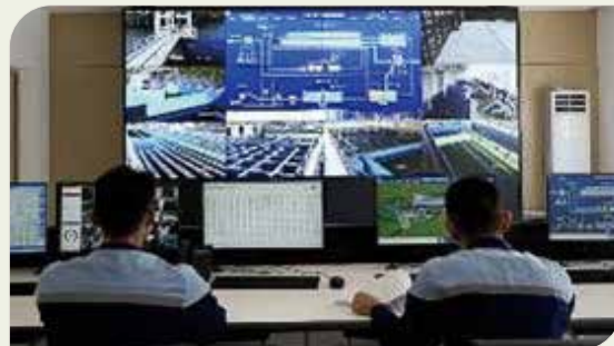
■ “Smart Water” Centralised Control Centre of Daluo Carbon Neutral Water Plant
